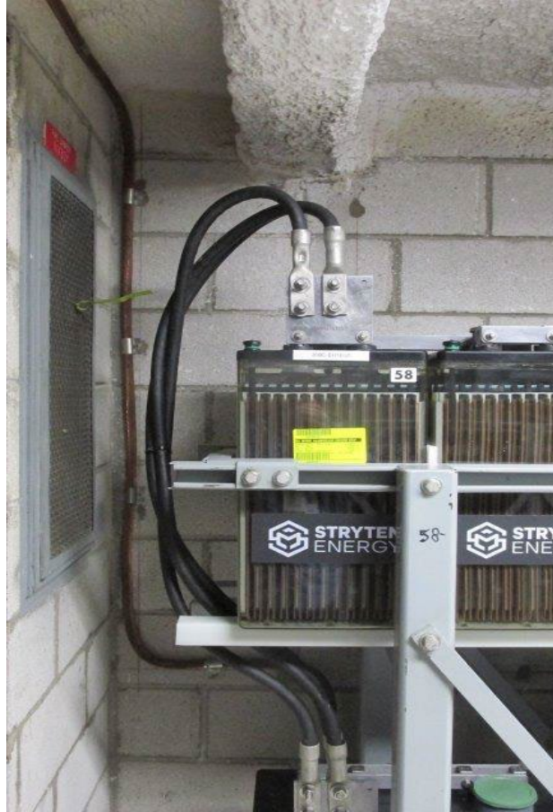
Figure 6. Unsupported Inter-Tier Cabling
