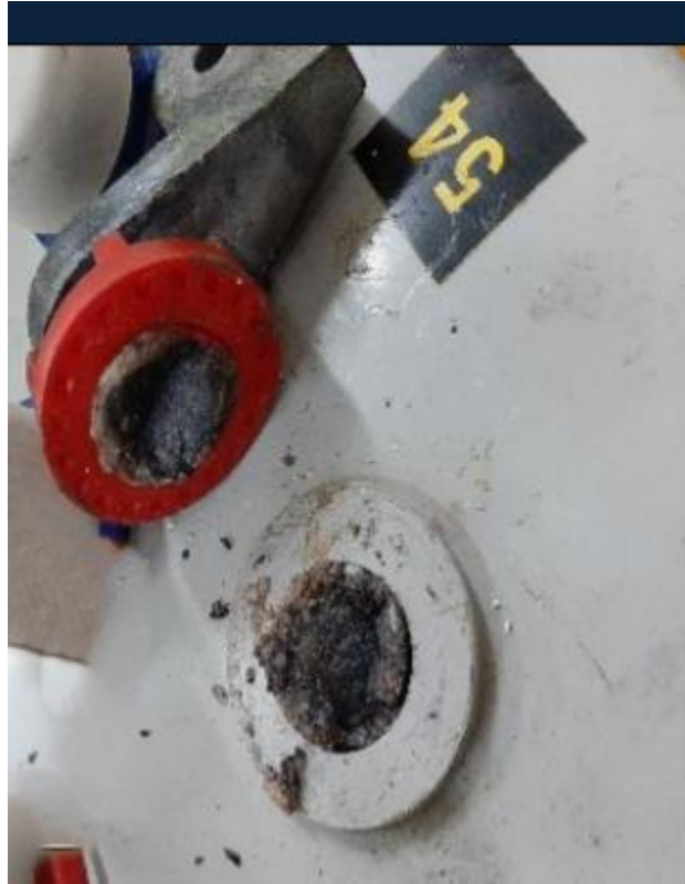
Figure 25 is the positive post in a very small cell that melted apart under its load. I previously identified this as a fragility issue and the result of “torque’ checking of the connection, but upon further study realized that it was a separation under load.
