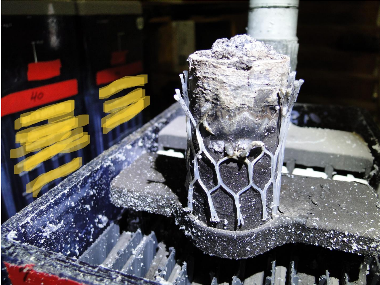
Figure 22 shows the positive post that melted apart when the power plant that it was supporting tripped offline. The battery failed open as soon as the inrush loads were applied. This battery had PASSED a capacity test at its published three-hour rate just 14 months prior to this event, and this cell was not the weakest cell in the battery string. It passed the test with over 100% capacity. The cell did not explode. This failure caused damage to the generator which took months to rebuild, and cost millions in repair costs and lost revenue.
