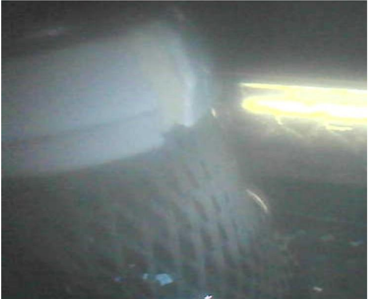
Figure 10 medium advanced expansion borescope capture
