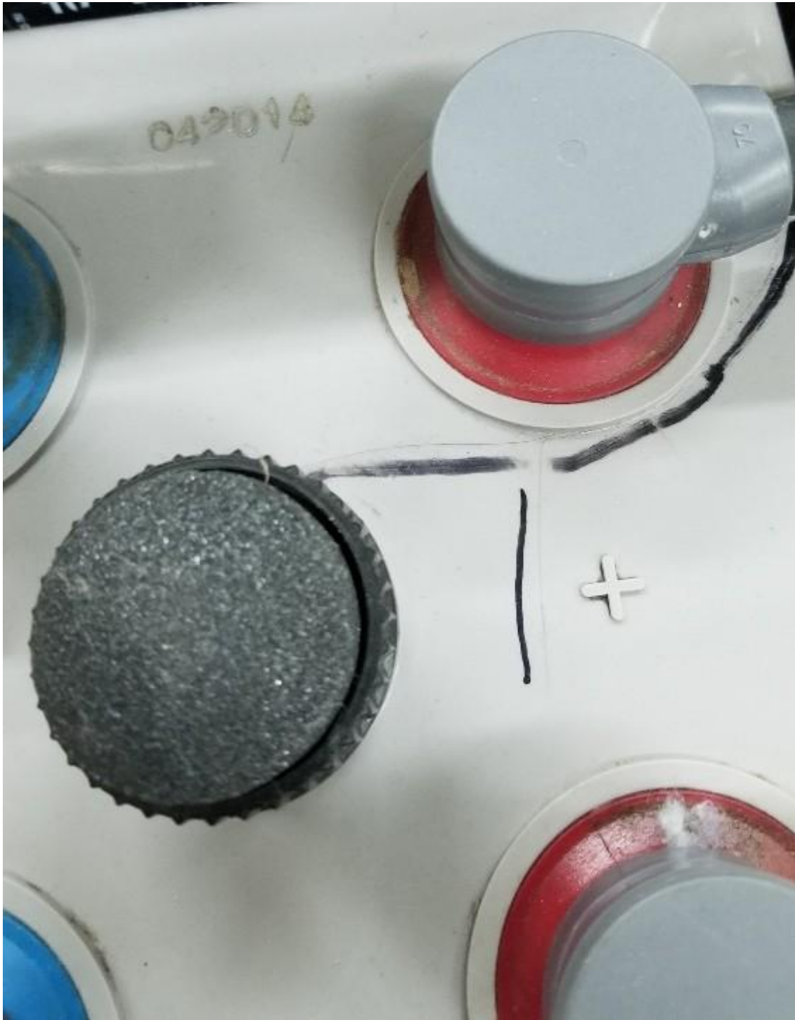
Figure 15 cover cracking proof of nodular corrosion presence
