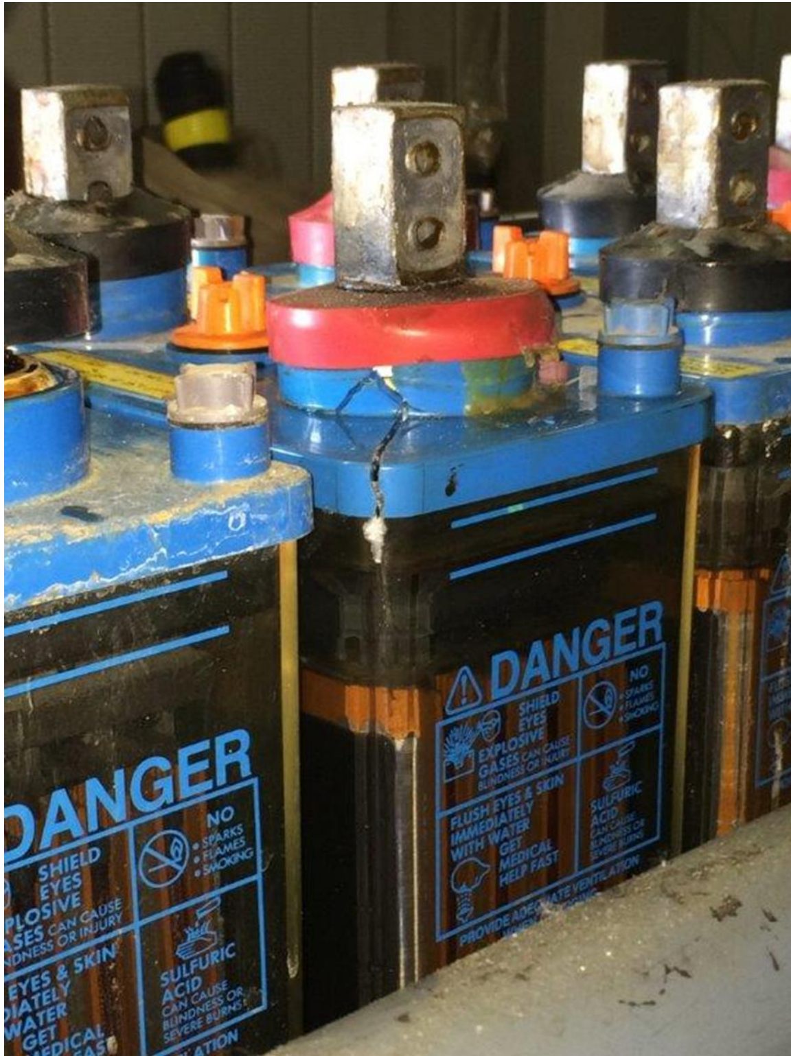
Figure 14 both creep corrosion and cover cracking due to nodular corrosion
