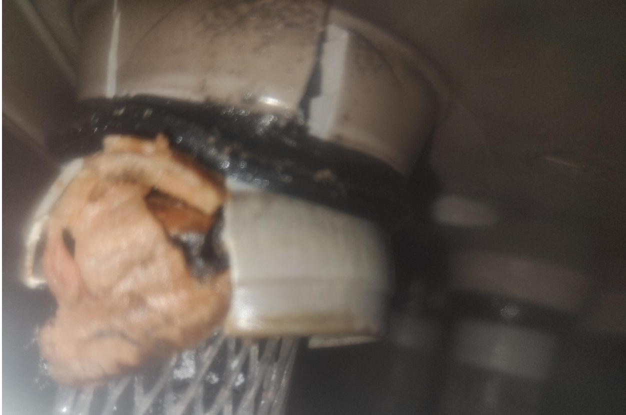
Figure 13 very advanced stage of degradation through jar wall capture – broken off plastic material was in electrolyte.
