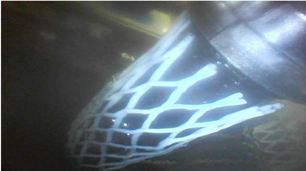
Figure 7 beginning of a crack in the side of positive post seal well wall
